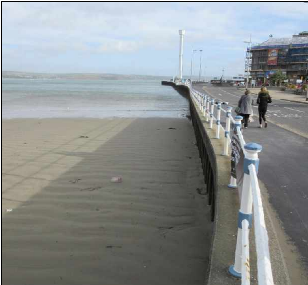
Figure 3.3 Typical existing 'Harbour Walls General' (Wall G, northern side of Pavilion Peninsula)
