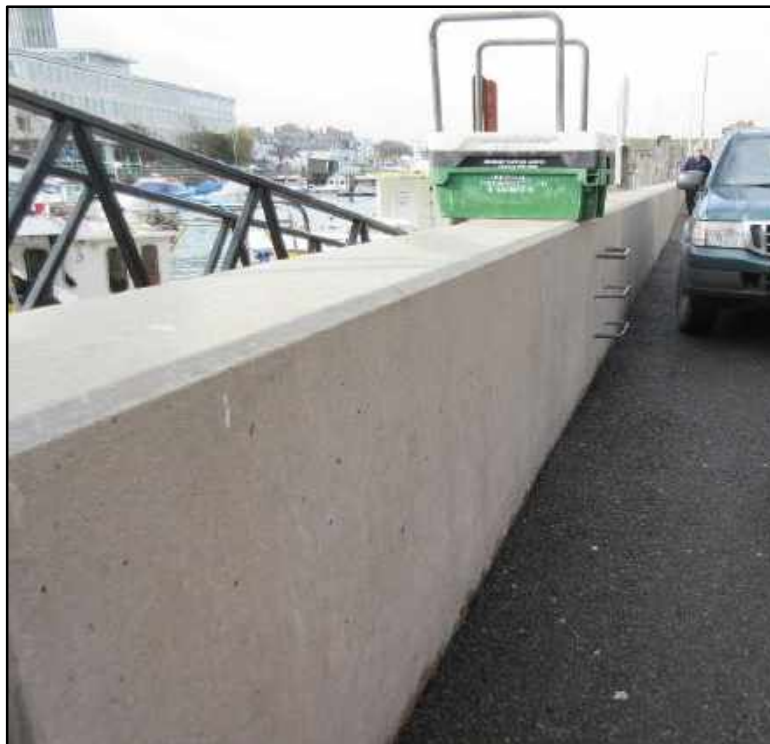
Figure 3.2 Typical existing 'Harbour Sea Defence Wall' (Wall 7, adjacent to Lifting Bridge abutment)
