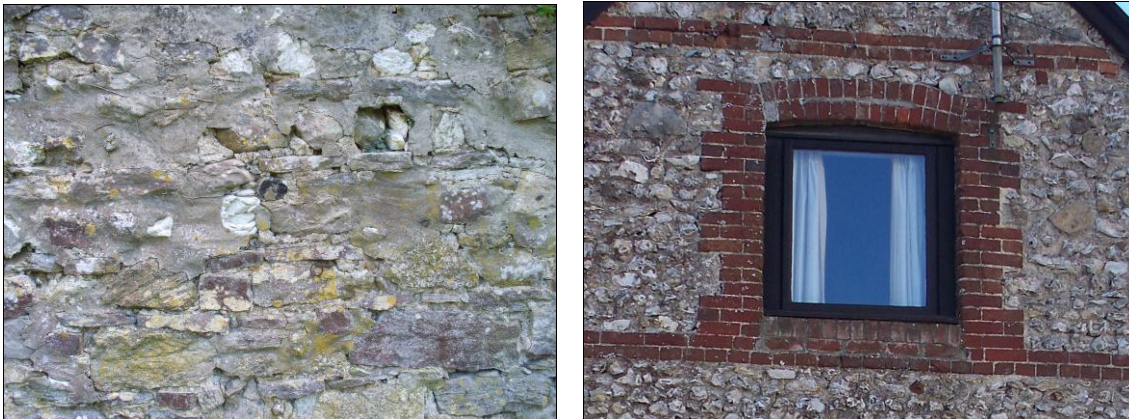
FIG. 10: Stone and brick. Left: Mixed rubble containing limestone, flint and chalk at Vicarage Farm. Right: Flint wall with brick dressings seen at the Granary.
