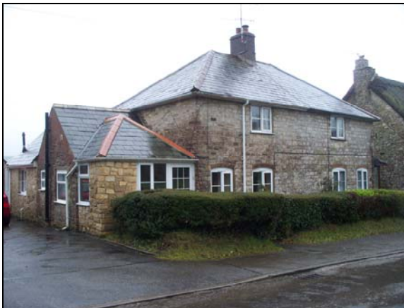
FIG. 6: Side extension. 14 Church Knowle. Here additions appear to have developed by accretion, the latest especially lacking harmony in terms of form, detail and execution.
