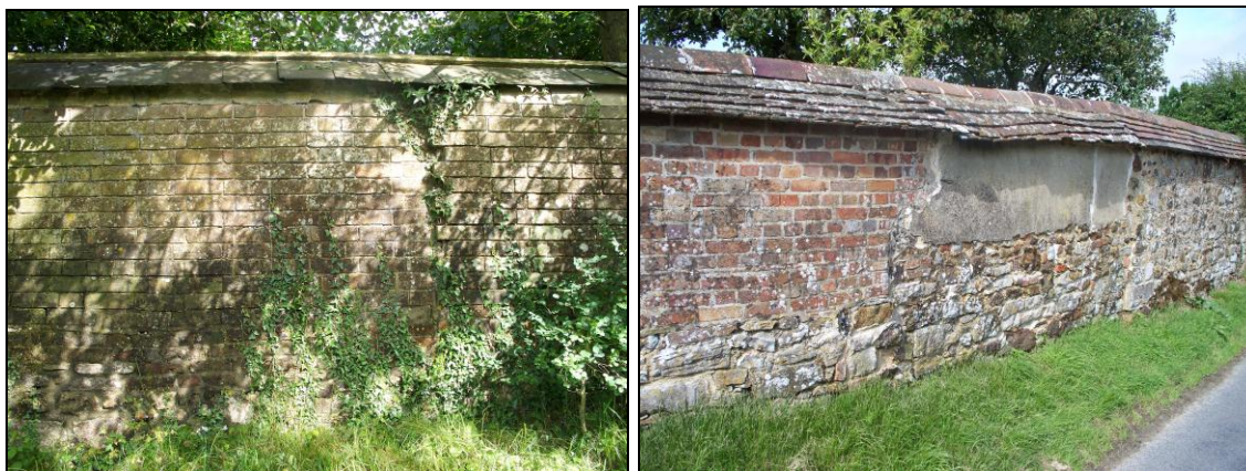
FIG. 5: Boundary walls. Left: Old Parsonage, pale brick with stone base and slate with stone ridge coping. Right: East Coombe Farm, wall containing elements of reused brick, stone and tile alongside cob, with a tiled coping.
