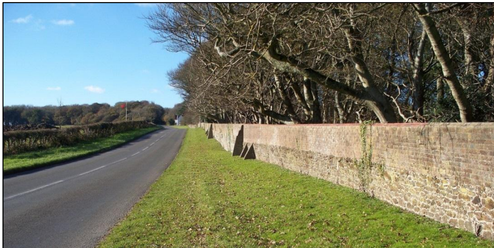
FIG. 8: The park wall. A major feature of enclosure within the conservation area, generally built on a masonry plinth (variously heathstone and or limestone with occasional flint), raised in brick adjacent to roads.
