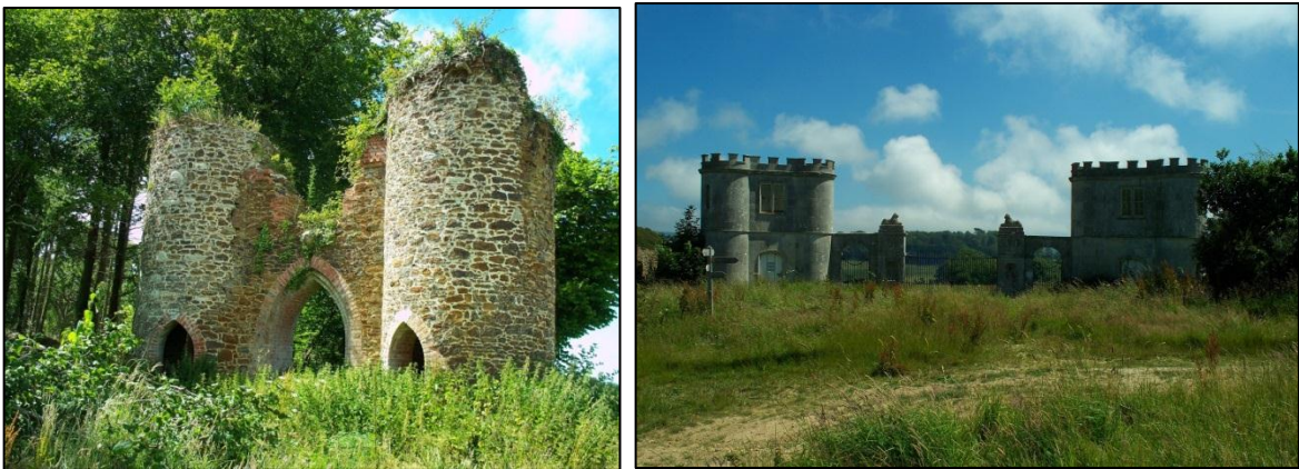
FIG. 12: Clare Towers and North Lodges. Clare Towers (right) is a ‘Gothic’ styled northern entrance to the park, whose heathstone construction is more visible since concealing ivy has been removed. This has also clearly exposed the poor condition of the structure. Higher quality Portland ashlar is used at North Lodges to the east (right), though flanking towers and walls are constructed from heathstone. This building is also in poor condition and on the Historic England ‘at risk’ register.
