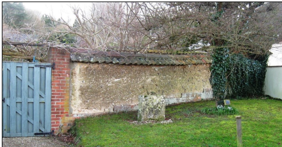
FIG. 20: Section of cob boundary wall, Briantspuddle. The protective coat of render appears to have fallen off or been removed. Note the pantile coping and brick plinth.
