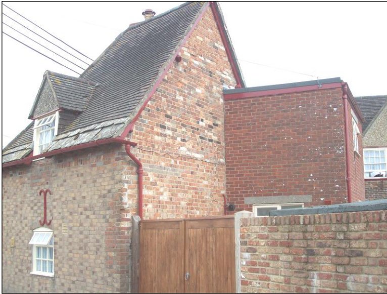
FIG. 7: Rear extension to Number 73, Corfe Road. This is insensitive in terms of its form, and the brick colour and bond employed.
