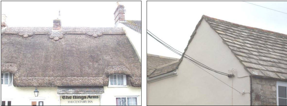
FIG. 9: Roofing. Left: the King's Arms. The ornamental 'block' ridge does not form part of the local tradition. Note also the use of ligger detailing just above the eaves, a feature which locally is generally restricted to the ridge. Right: Nos. 65 and 67. The stone roof is pointed and the rear extension coated with reconstituted stone.
