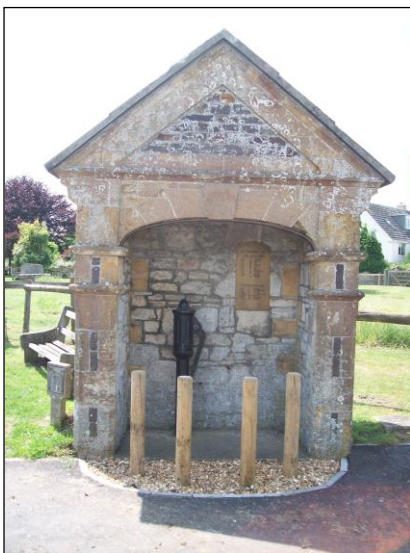
FIG. 13: The Pump House. These wooden posts restrict access and communication with the heritage asset while visually detracting from its significance.
