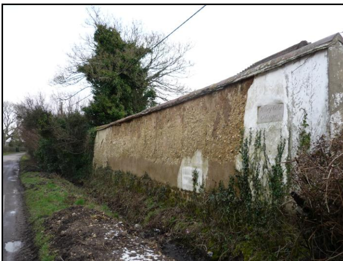
FIG. 13: This cob wall in Bindon Lane stands on a brick plinth and has a tiled roof to protect it from rainwater. Unfortunately this particular example is in a state of disrepair.
