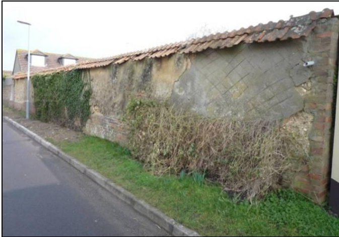
FIG. 27: Cob wall on the High Street in poor condition. Cement render used to repair the surface is causing further harm.
