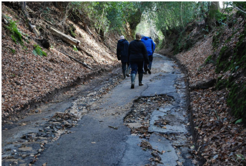
Fig. 9. Damage to sunken lane, Hammer Lane, Iping, West Sussex.
