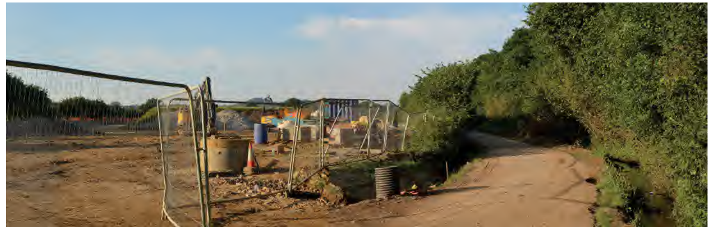
View north from the south-eastern corner of the western parcel showing part of the site and Watery Lane
